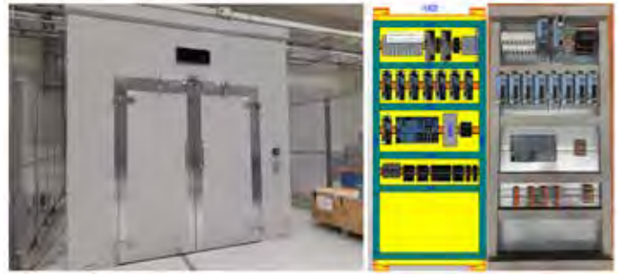
Figure 2.3.4 Remote laser system enclosure (L) and control cabinet build (R)
